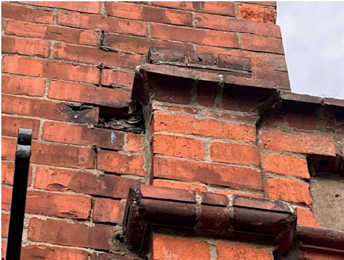
Town hall leak
