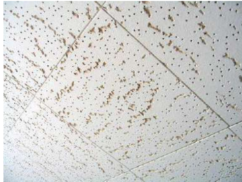
Asbestos containing ceiling tiles
