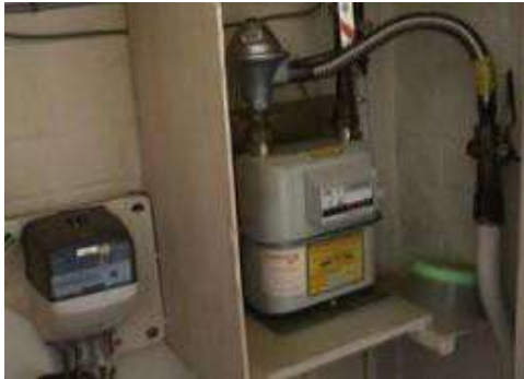
Asbestos panelling around a gas meter
