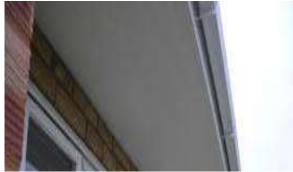
Pieces of Asbestos Insulating Board (AIB)
