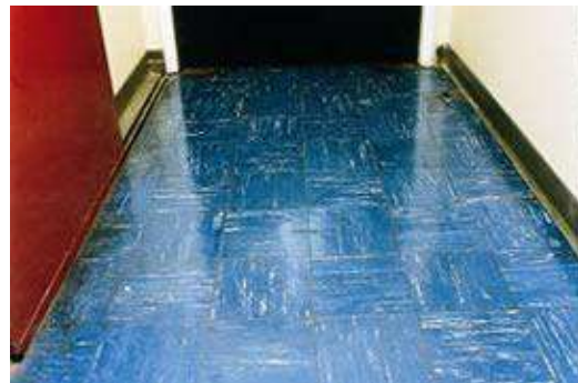
Asbestos containing floor tiles in a corridor
