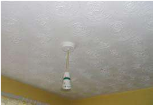
Asbestos textured coating
